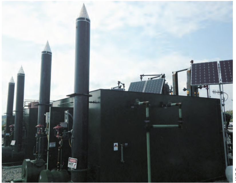
Equipment at a gas well.
